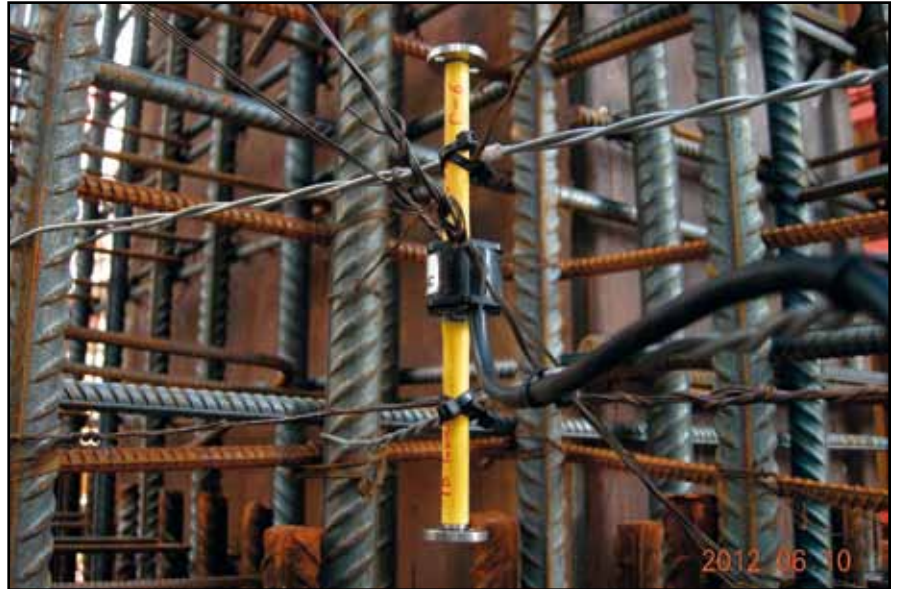
Figure 11.5 Vibrating-wire strain gauges.
