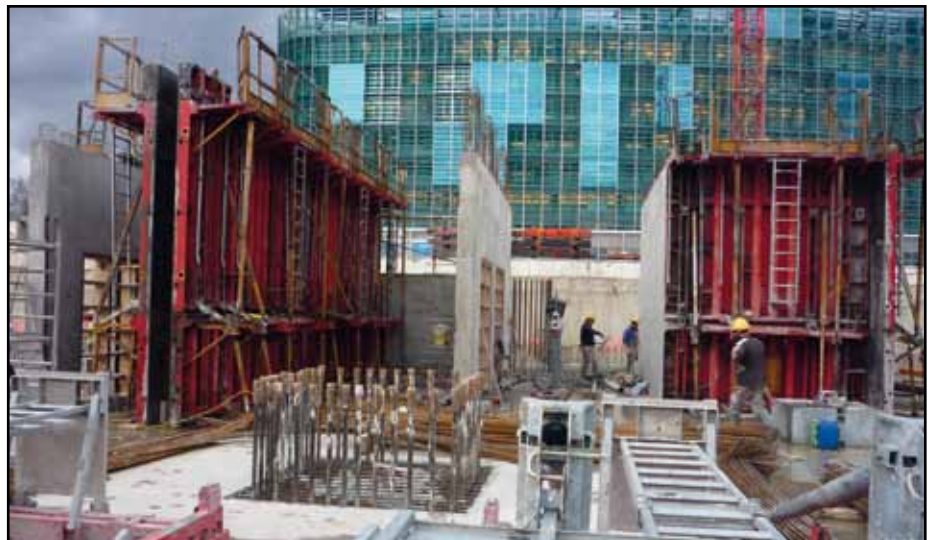
Figure 7.1 Loading from construction materials and activities may be the dominant imposed load.
