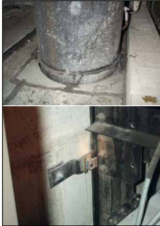
Figure 11.2 Bond failure between sealant and slab (upper) and scrape in lift guide rail (lower) due to downward movement of the building structure (90 mm) relative to non-structural elements (Bast et al. 2003) [25] .
