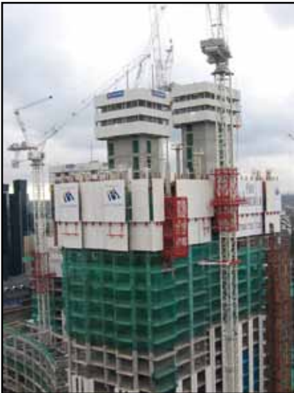
Figure 6.7 Hydraulic self-climbing enclosure systems for core and slab construction. Photo: Laing O'Rourke Plc
