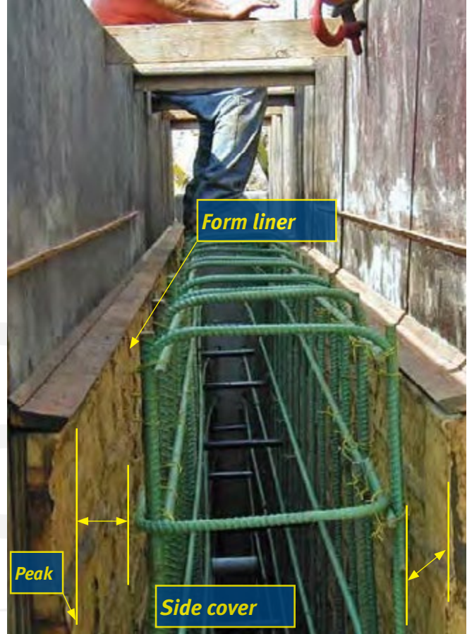
Fig. 5: View of formwork, formliner, and reinforcing showing side cover measured to the peak of the formliner
