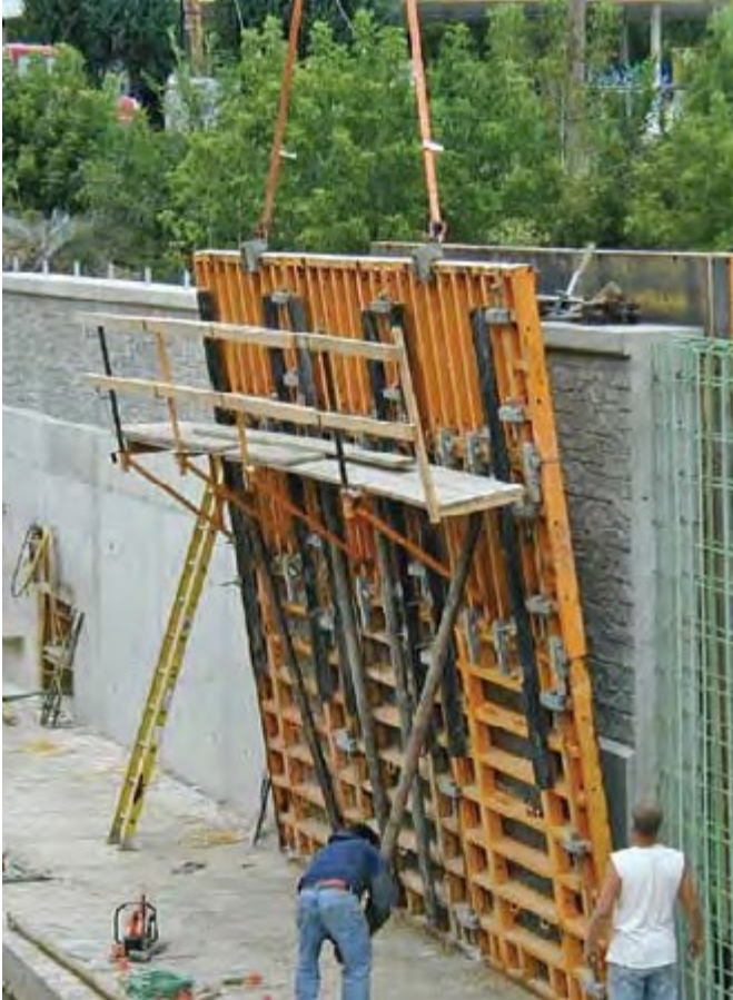
Fig. 4: Concrete wall cast using a formliner designed to simulate a masonry wall (photo courtesy of Gewalt Hamilton Associates)
