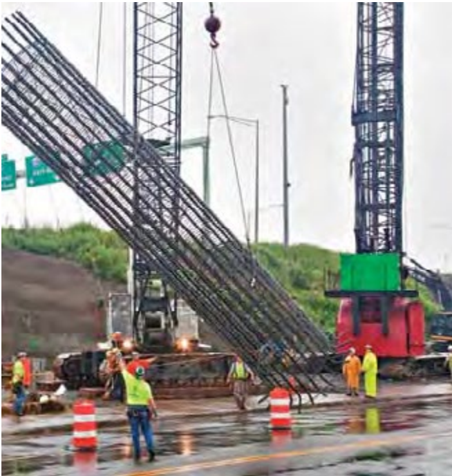
Fig. 7: A well-braced drilled shaft cage is picked with minimal distortion (photo courtesy of Dimension Fabricators, Inc.)
