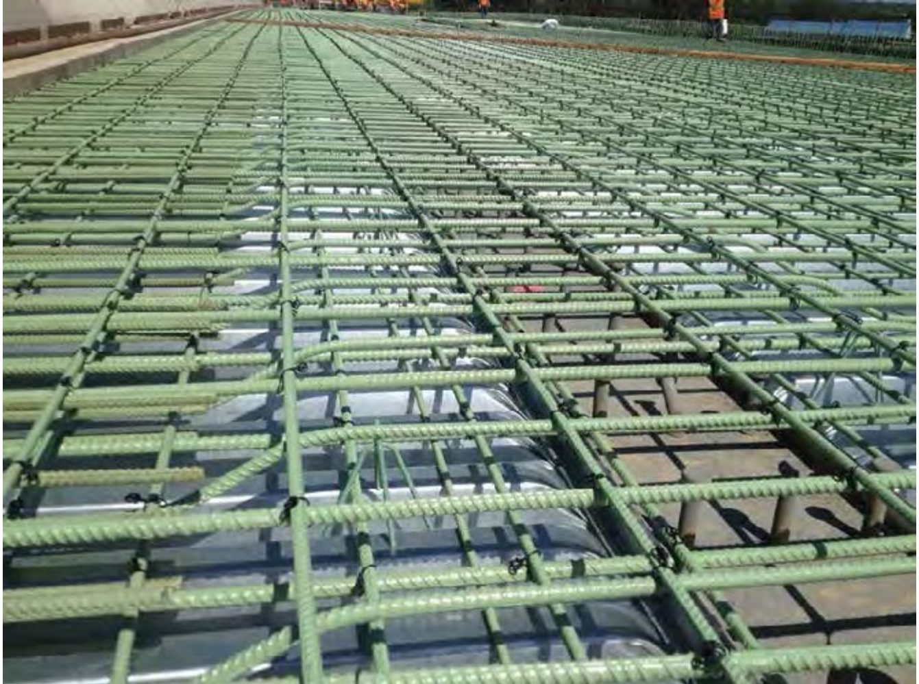
Fig. 3: Example of truss bars used in a bridge deck. To maintain cover tolerance (normally +0 in. (+0 mm) for bridge decks), top horizontal segments may need to be shifted slightly relative to the bottom horizontal segments
