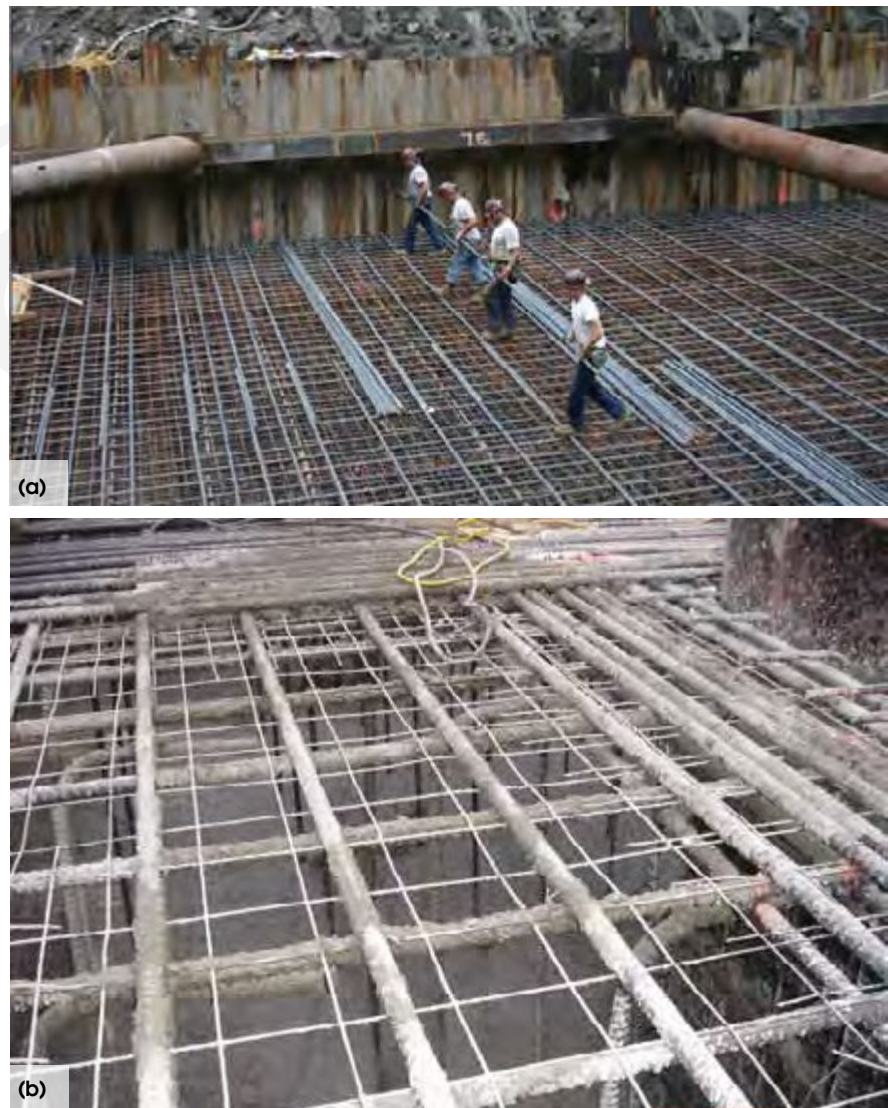
Fig. 7: WWR placed between the top reinforcing bar layers allows the workers to safely walk on the mat before and during concrete placement: (a) Trump Tower, Chicago, IL; and (b) Roosevelt University, Chicago, IL (photos courtesy of Jack Gibbons, CRSI)
